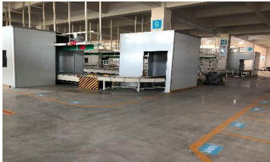
Air Conditioner Plant View
