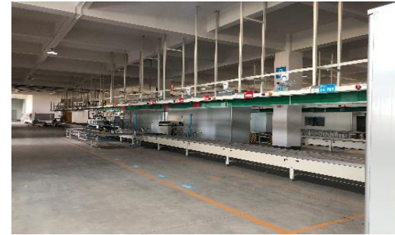
Air Conditioner Plant View
