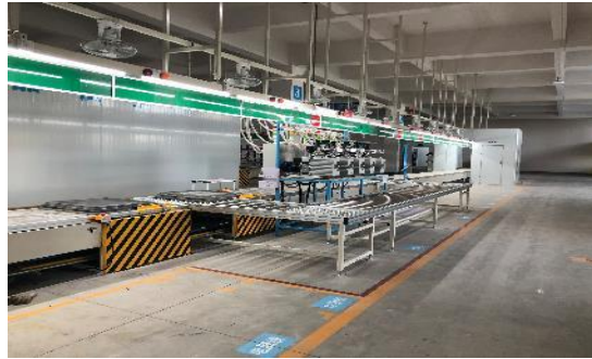
Air Conditioner Plant View
